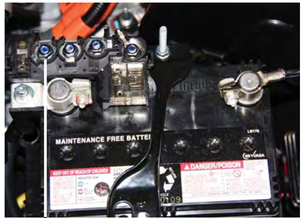
DC to DC Converter Cable Connection
