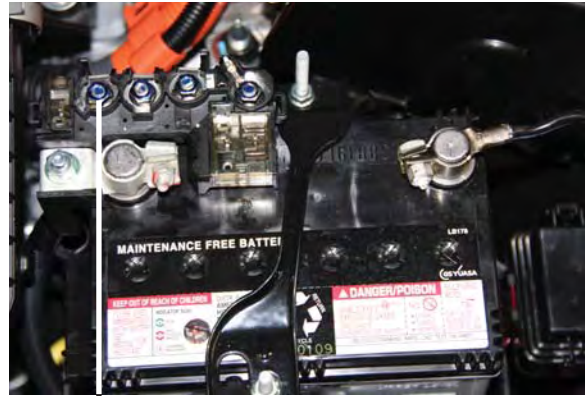
DC to DC Converter Cable Connection
