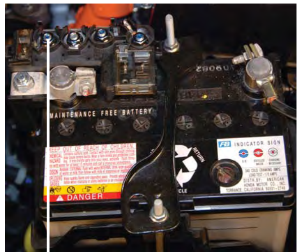
DC to DC Converter Cable Connection
