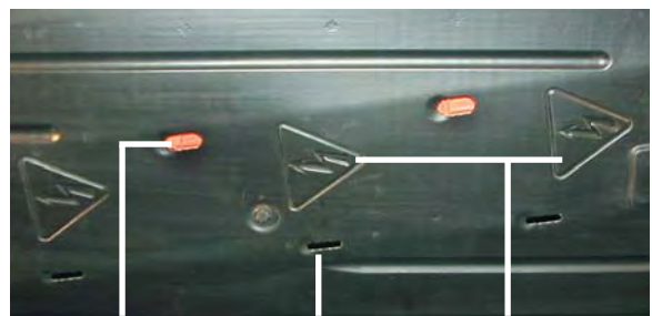
High-Voltage Cable Visible
