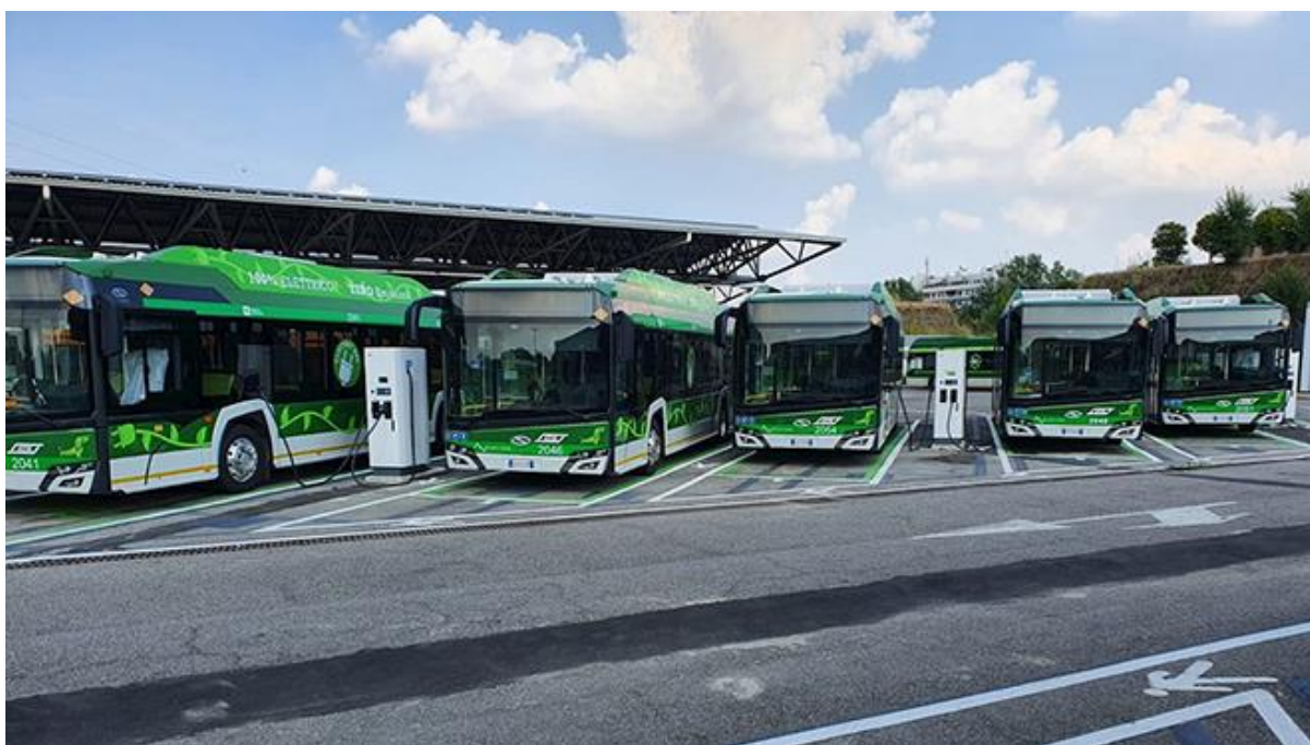
Photo 4: Electric Bus Charging Bay
