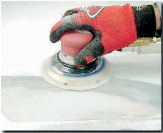
J-6 The finish around the repair area can be featheredged with a dual-action sander.
