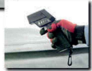
C-7 LEFT: This panel is heated with a torch during the straightening process. RIGHT: A non-contact thermometer is used to monitor the temperature.
